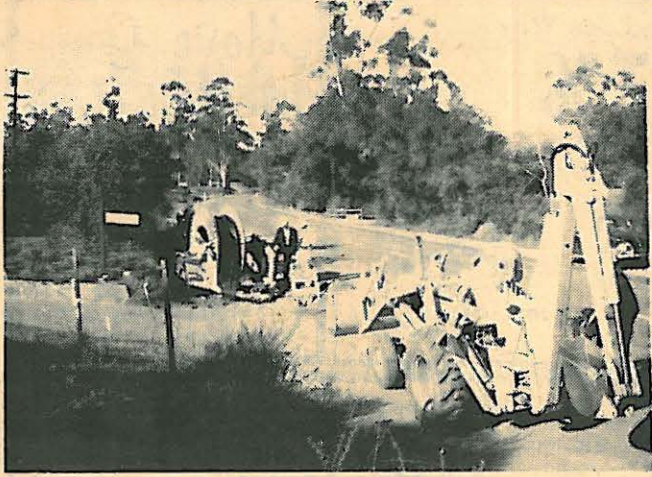
MORE PROGRESS IN THE EAST COUNTY FOOTHILLS AS THE TELEPHONE COMPANY INSTALLS NEW LINES IN ALPINE ON ARNOLD WAY. (Echo-Sun Photo)
